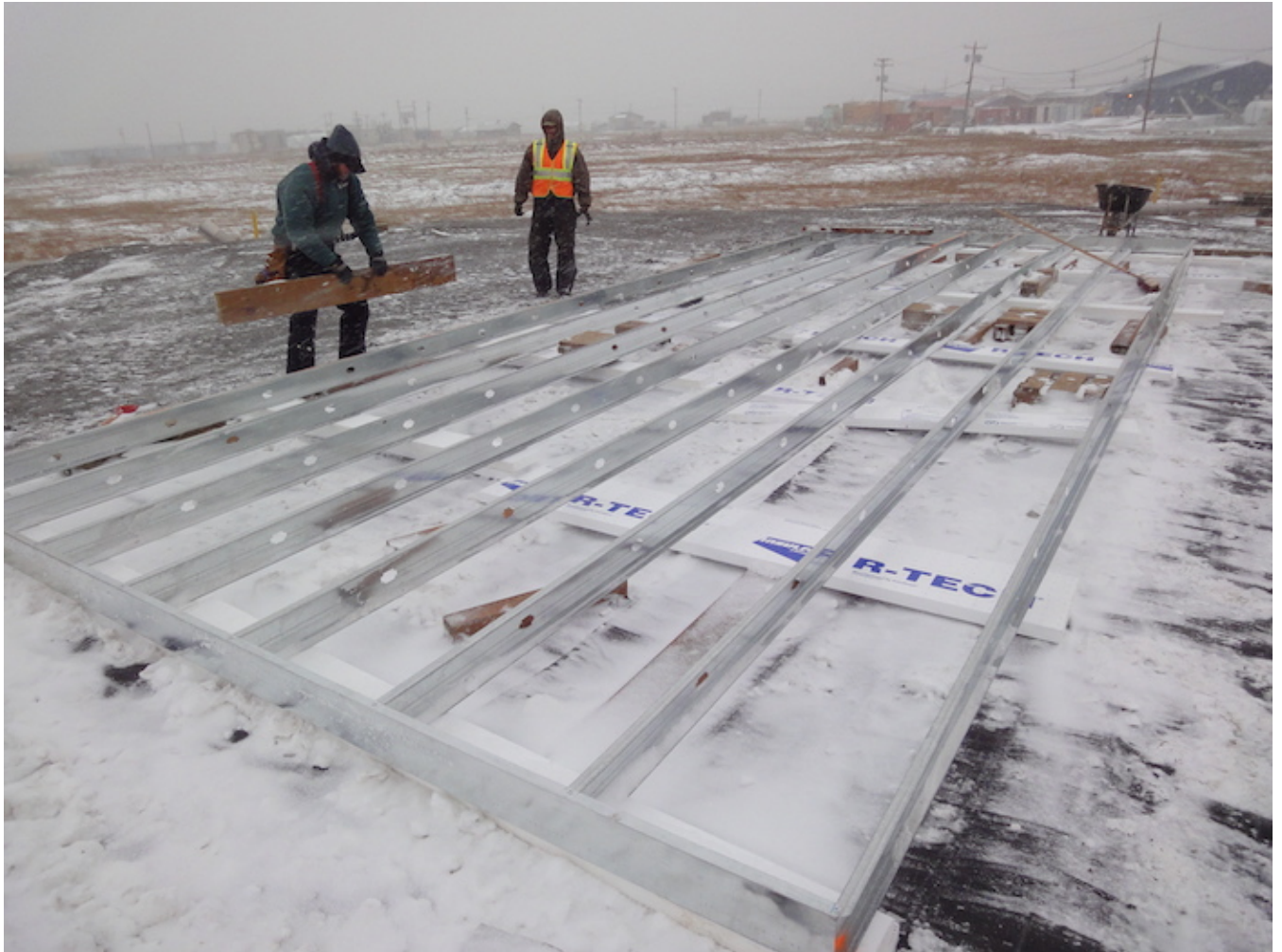
Figure 3. CCHRC partnered with the Yup'ik community of Quinhagak in 2010 to build a super-insulated home that could withstand the cold, wet climate of the Bering Sea Village. Photo Courtesy of CCHRC.
